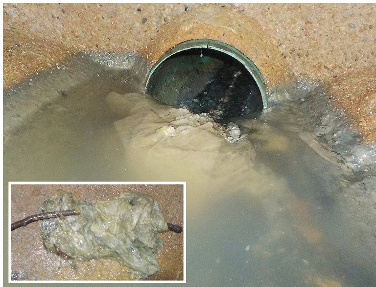
Figure 3. Smart sewer technologies identify developing blockages before a problem arises
