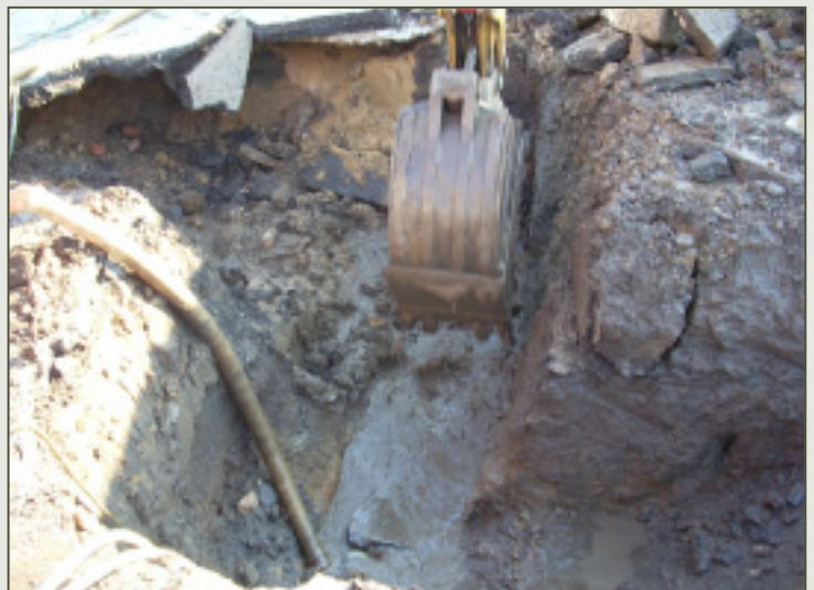
Excavation conducted to expose the leak for repair while leaking water was being pumped out.
