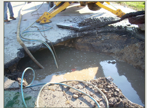
Excavation of a leak found that did not come to surface. The erosion of the ground under the asphalt could have caused a failure of the road surface at any time.
