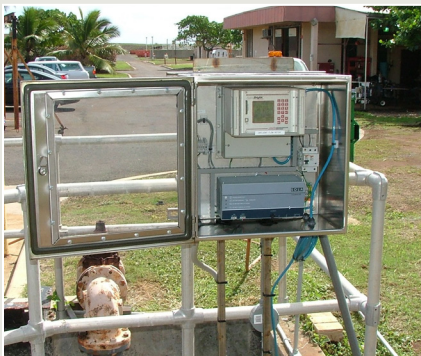
Cross correlation depth/velocity meter interface shown here after mounting and hookup of sensor and SCADA wiring.
