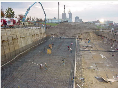
A 3-million-gallon underground storage tank, completed in the Fall of 2004, has significantly reduced the raw sewage overflows into the White River in downtown Indianapolis. This tank is part of the city's long-term plan to reduce sewage overflows and restore Indianapolis rivers and streams.
