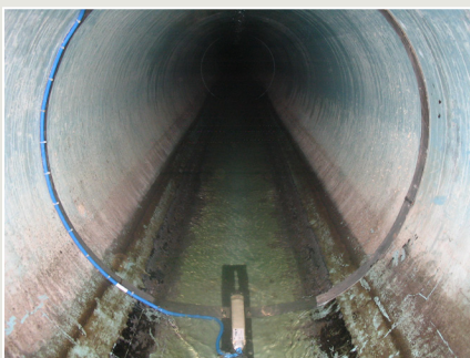
Cross correlation type depth/velocity sensor installed on stainless steel mounting ring in plant's influent pipe.
