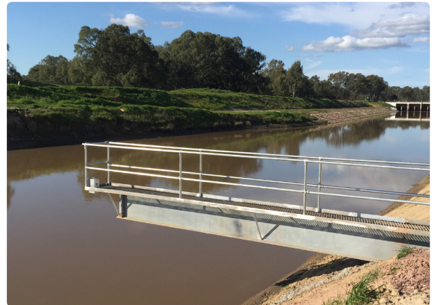
Coleambally Channel ACCUSONIC Installation
