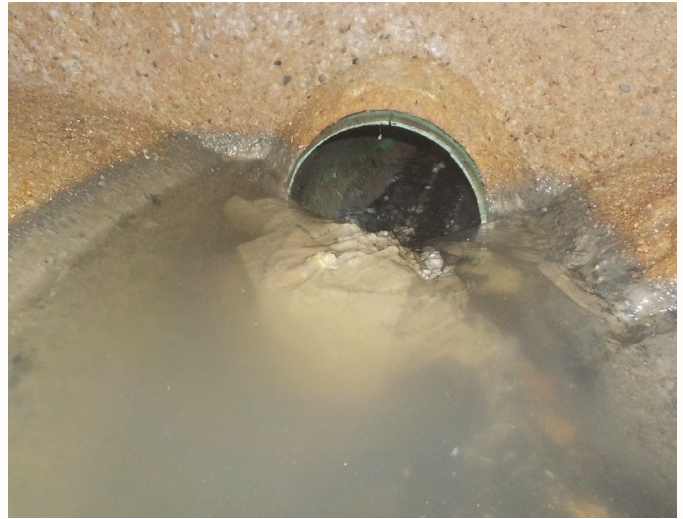
Stick blocking outlet pipe resulting in ragging.
