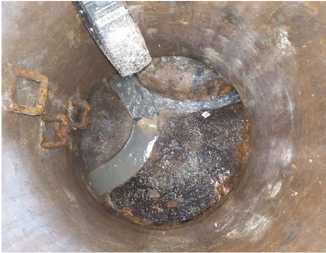
Grease blockage observed in manhole channel.
