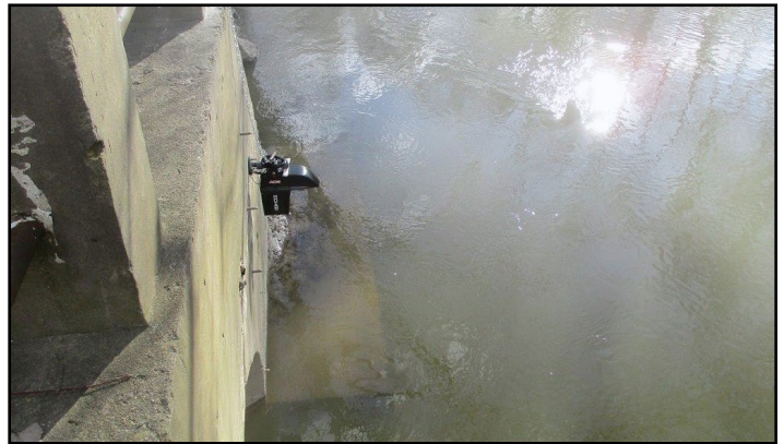
Image 3: ADS ECHO installed on a bridge for river level monitoring of the Detroit River
