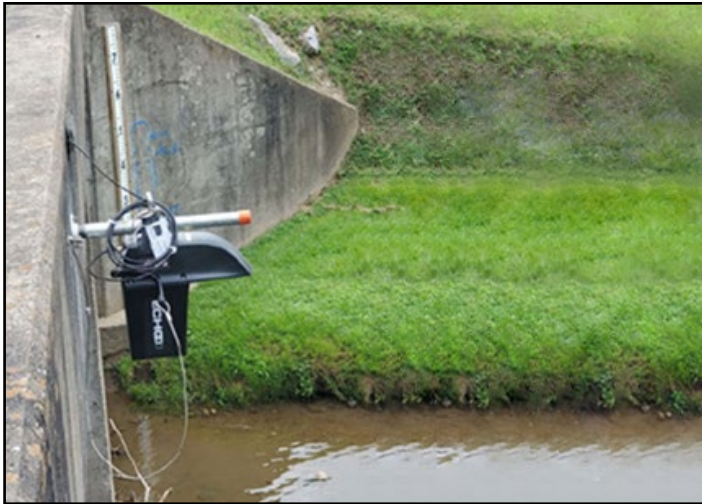
Image 4: ADS ECHO level monitor installed on a bridge
