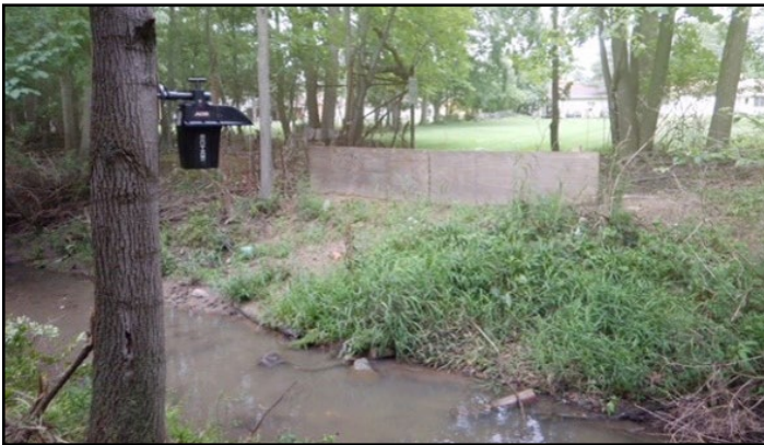
Image 2: ADS ECHO installed for stream monitoring to avoid park flooding
