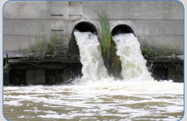
CSOs can be a major source of water pollution in communities served by Combined Sewer Systems. These systems serve over 43 million people in approximately 1,100 communities nationwide.
