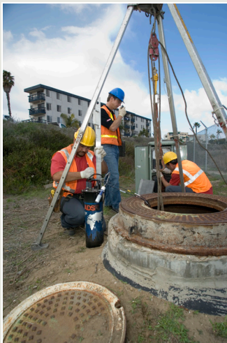
Wireless communications were connected to flow monitors to deliver real-time flow and alarming data.
