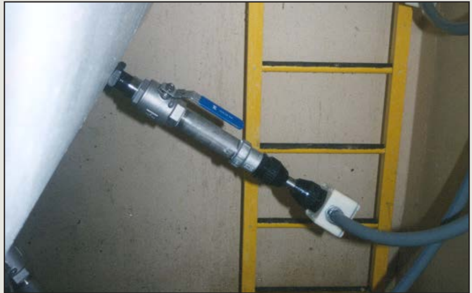
Model 7656/7655 Transducer/Feedthrough Installed in Combined Sewer
