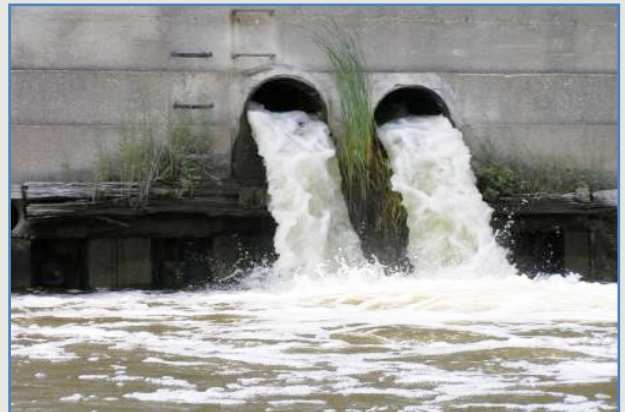
CSOs can be a major source of water pollution in communities served by Combined Sewer Systems. These systems serve over 43 million people in approximately 1,100 communities nationwide.
